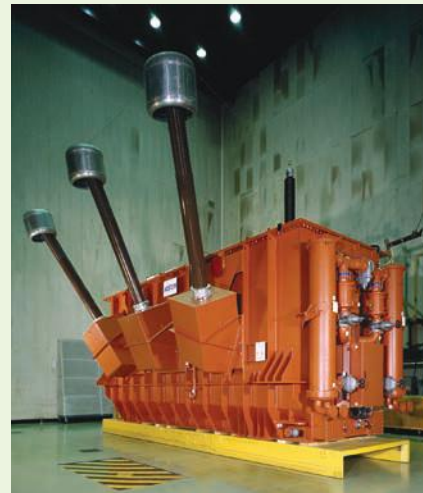
Figure 44.5 Step-up transformers at a power station
